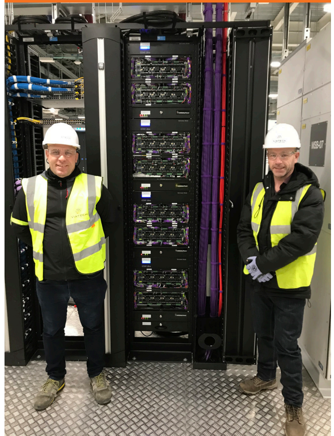
Viatch's VIA-COMP® cables installed into the Meta Datacenter, Clonlee Ireland
